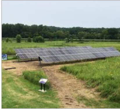
Freestanding solar array at Hurstville Interpretive Center. Photo Credit: Jackson County Energy District website
